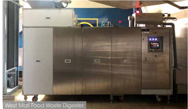
West Mall Food Waste Digester
